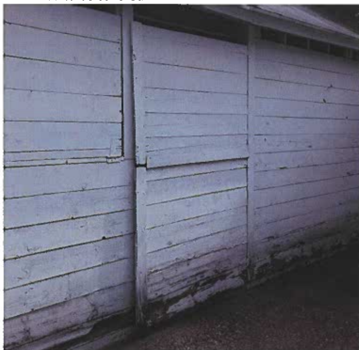
Rotted siding, door needs to be replaced, & pigeon openings that need to be covered.
