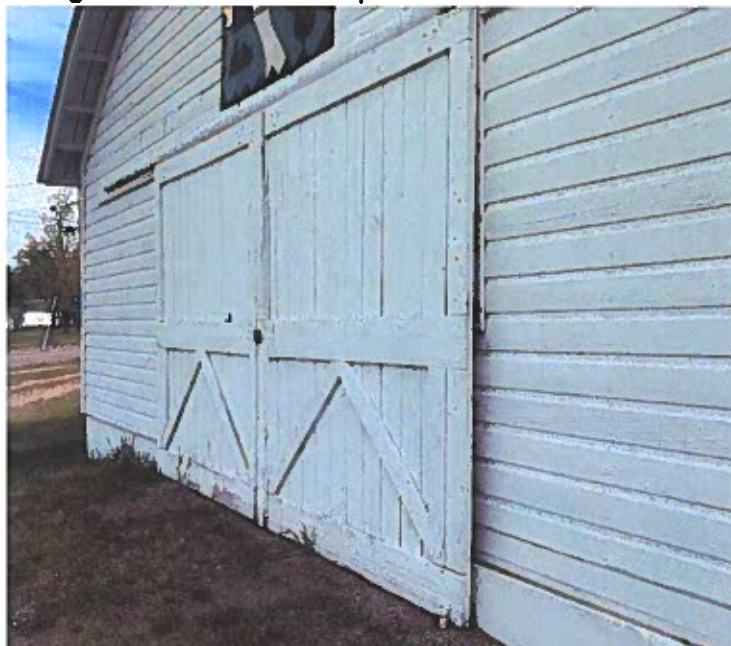
Sliding door that should be replaced.
