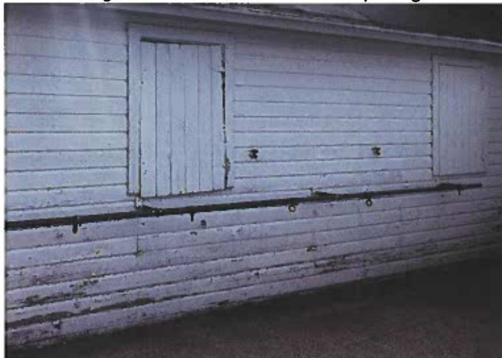
Rotted siding & window cover that needs replacing.
