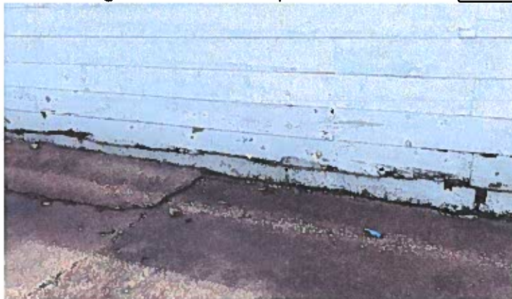
Rotted siding that needs to be replaced.
