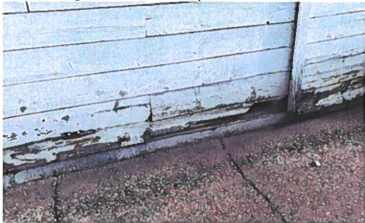
Rotted siding that needs to be replaced.
